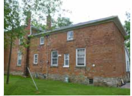
This photograph shows exposed foundation above grade being maintained as part of the building elevation. (Source: ERA)
