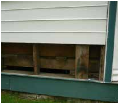
This project involved carefully removing part of the exterior wall in order to expose the interior structure and understand how to properly reinstate the exterior siding. (Source: ERA)
