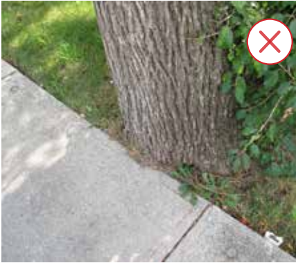
Widening of the roadway has encroached on this tree's root system. (Source: ERA)
