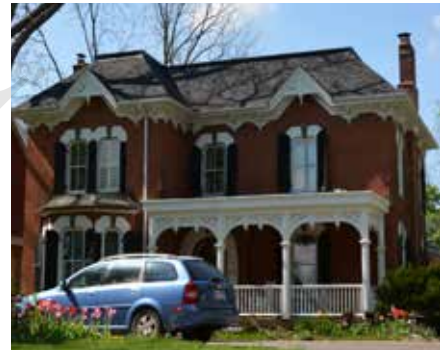
Original roof features shown here, like the cornice, brackets and fascia along the roof's edge, and the spindlework within the small gables, are integral in conveying this house's architectural character. (Source: ERA)
