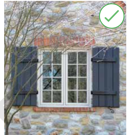
This photo shows operable storm shutters that are appropriately sized. (Source: City of Brampton)
