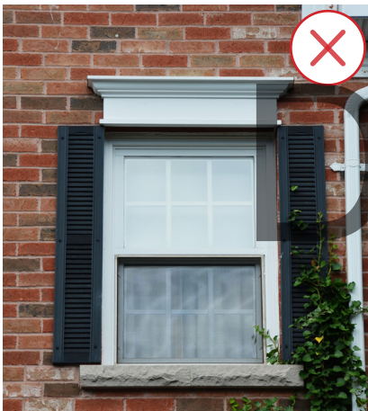
This photo shows storm shutters that are not appropriately sized for the window (Source: City of Brampton)
