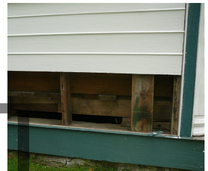
This project involved carefully removing part of the exterior wall in order to expose the interior structure and understand how to properly reinstate the exterior siding. (Source: ERA)
