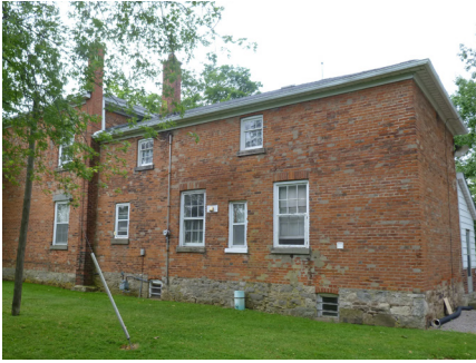
This photograph shows exposed foundation above grade being maintained as part of the building elevation. (Source: ERA)
