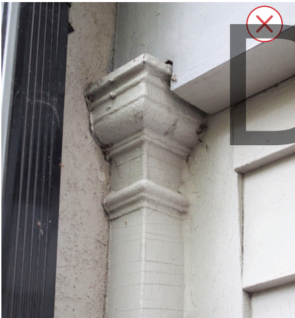
In this case, the decorative element was not well considered when making changes to the building. As a result, it was partly obscured. This should be avoided. (Source: ERA)
