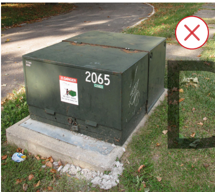
Installation of public utilities on Main Street South impacts the heritage character of the streetscape. (Source: ERA)
