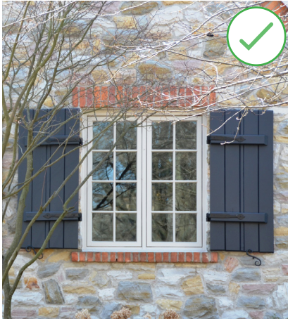
This photo shows operable storm shutters that are appropriately sized. (Source: City of Brampton)
