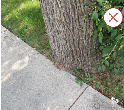
Widening of the roadway has encroached on this tree's root system. (Source: ERA)
