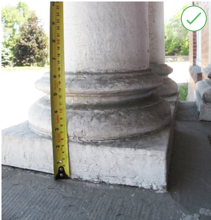
Completing detailed measurements of this column base was the first step in conserving this column. (Source: ERA)
