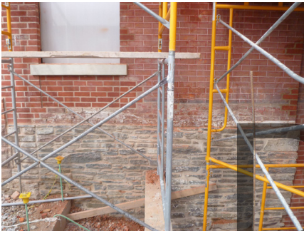
Ensure that contributing finishes and textures of foundations are maintained . Repair or replacement should match the historic texture and finishes (Source: ERA)
